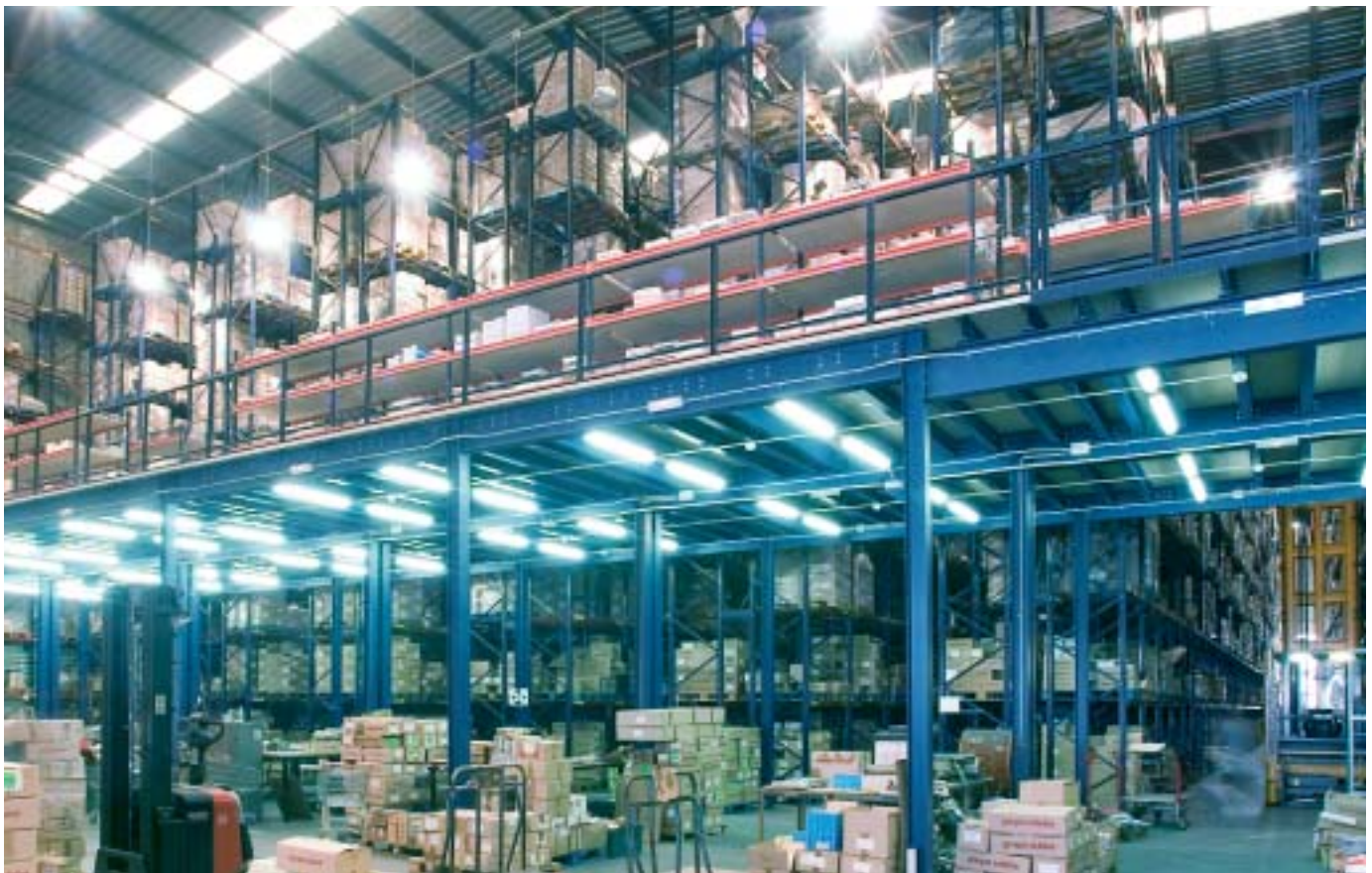
In the bottom part of the mezzanine, bulky products are stored while shelving for storing small and medium-sized goods has been fitted in the top part.
