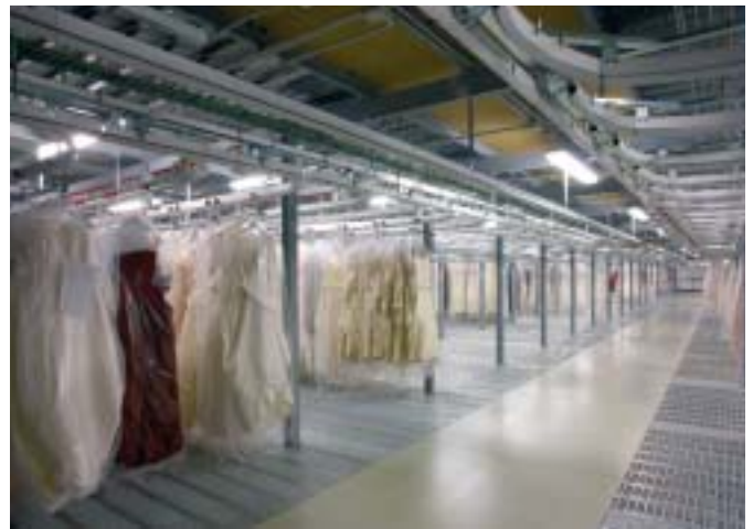
The mezzanine, in this case with several levels, is used as a classification and storage area for hanging items of clothing. The structure itself supports the elements required for the movement of the clothing trolleys.
